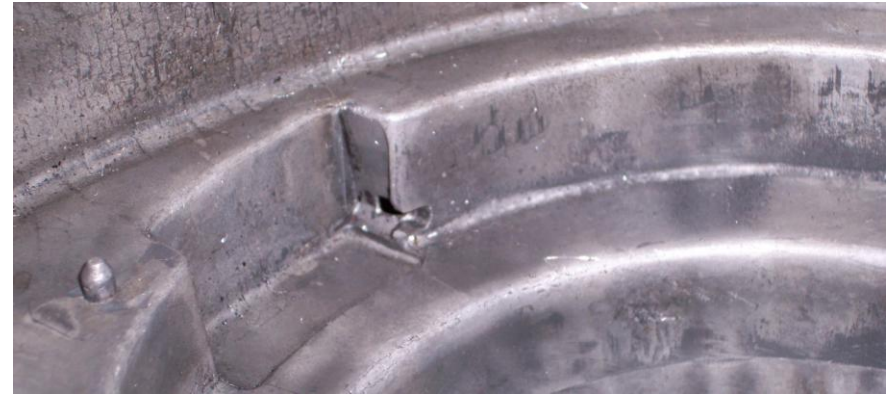
Pump pocket in need of repair
